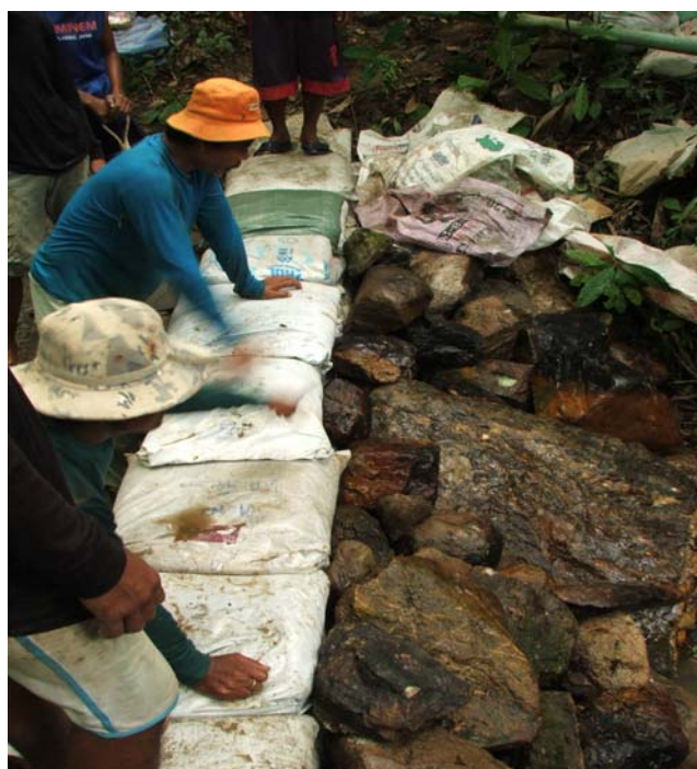
Villagers in Sanga-U, Koh Lanta, Thailand construct a check dam to retain rainwater
